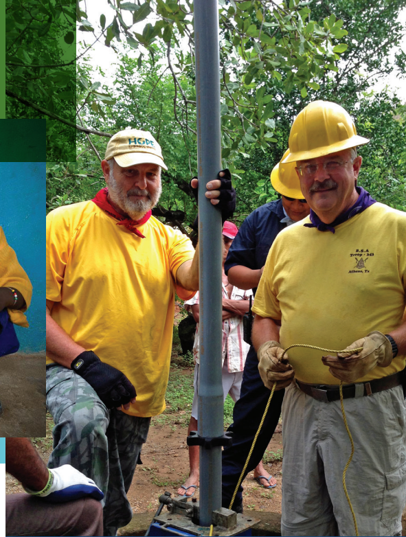
Bruce Hinds (left) and Ted Mettetal work to recover a well pump in Nicaragua.
